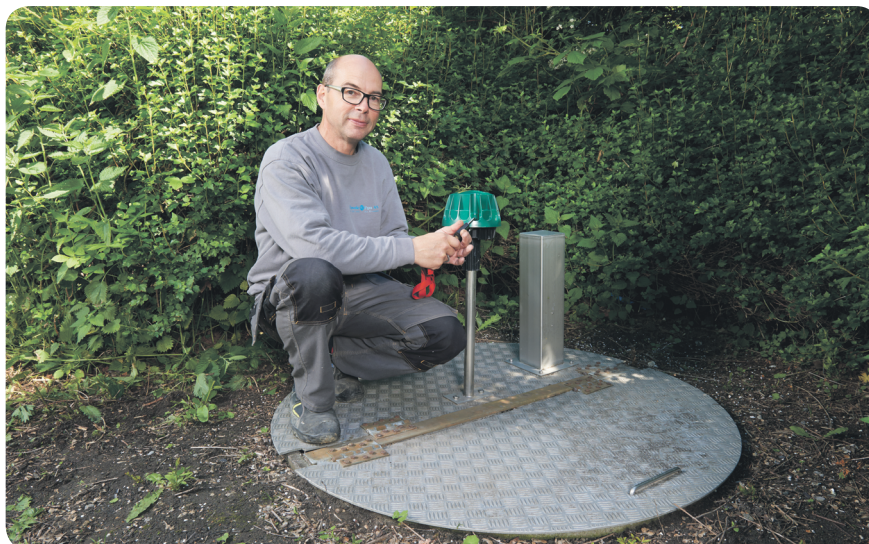
Carsten Kock showing the secured Chatter device behind the local community hall, the Chatter runs a monitoring routine every fifth minute. The Chatter device is powered via the sewer well.
